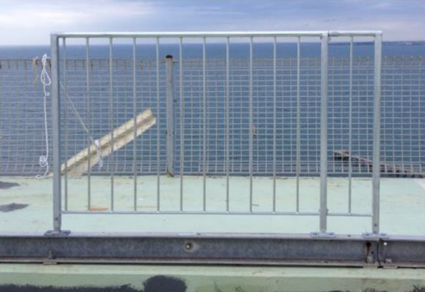
2014 Balustrade prototype on BMU beam. Rope access points installed in BMU beam.
